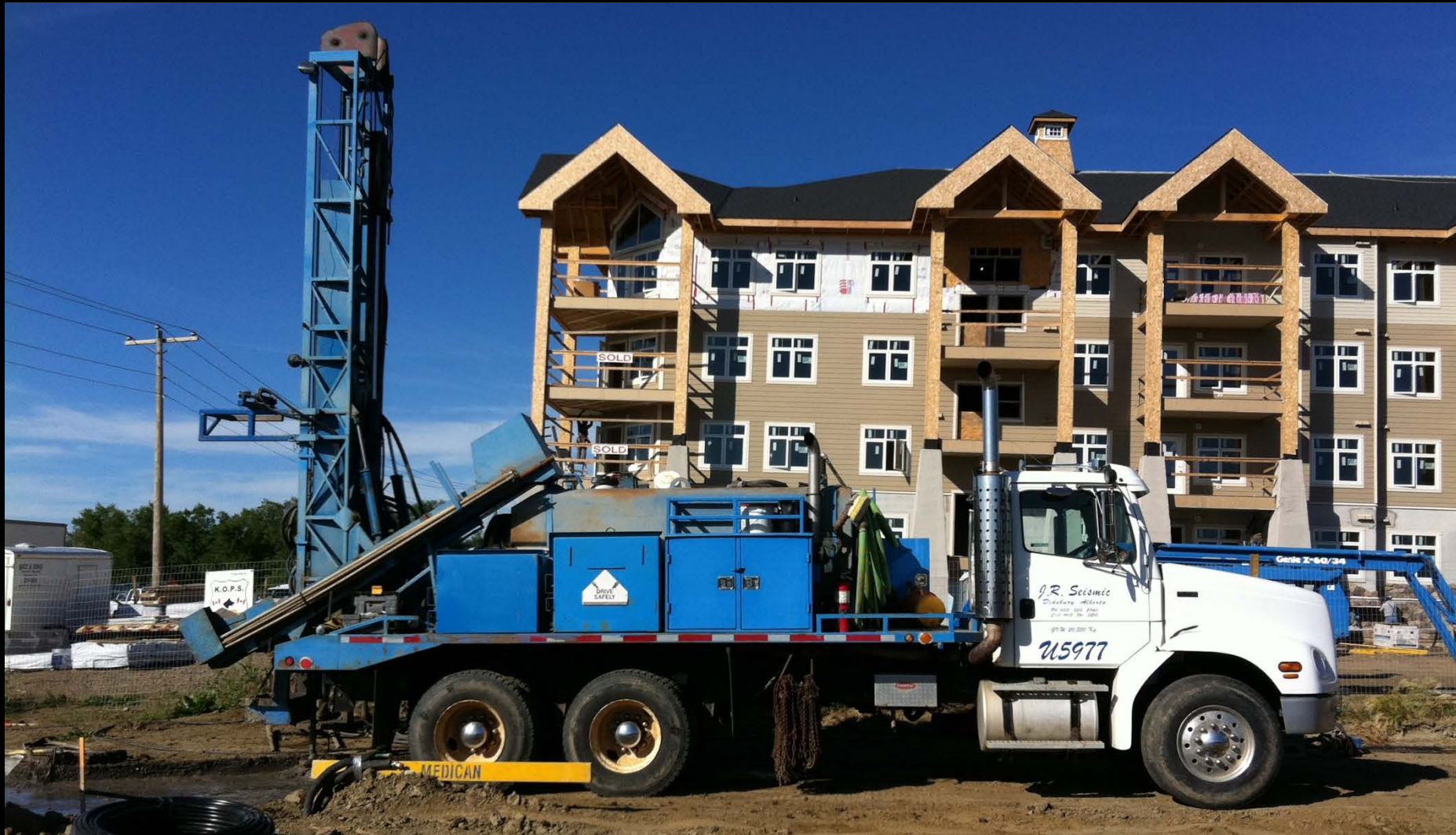
JR Seismic and Energy Smart Installing the System at the direction of Tim Padfield
